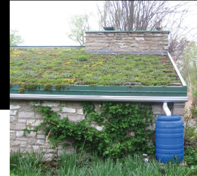
Civic Garden Center Roof, Cincinnati, USA Example rain event (12mm)
